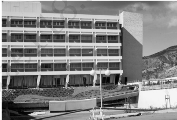
FIGURE 13.5 Permanent offset of weak first story due to discontinued wall, Olive View Hospital, 1971 San Fernando earthquake. (Photograph by K. Steinbrugge, used with permission from the National Information Service for Earthquake Engineering, University of California, Berkeley.)
