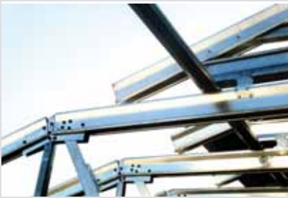
Cap truss installed on top of base truss. Note continuous bracing on top chord of base truss and connection clip.
